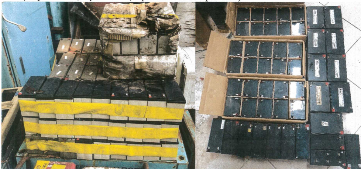
BATTERIES (22 pcs 3SMF, 5 pcs 2SMF, 9 pcs HFR & 130 pcs 12v )
